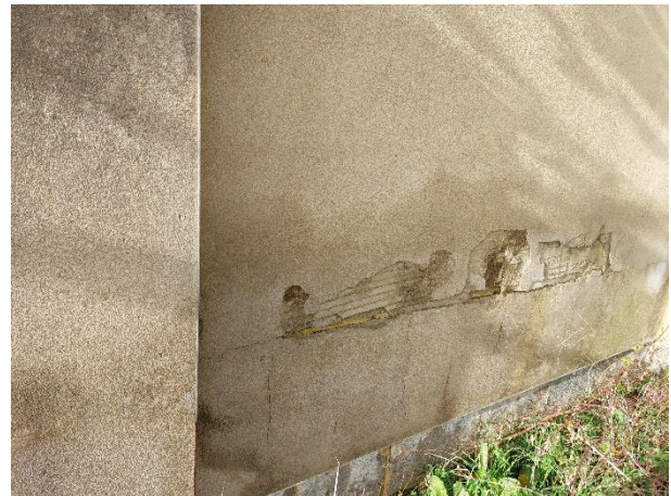
Damaged render, block below sealed
